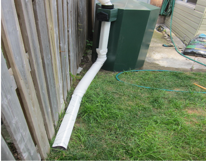
Figure 3.2: Installed rain barrel and overflow/bypass drainage at Hastings Ave.
